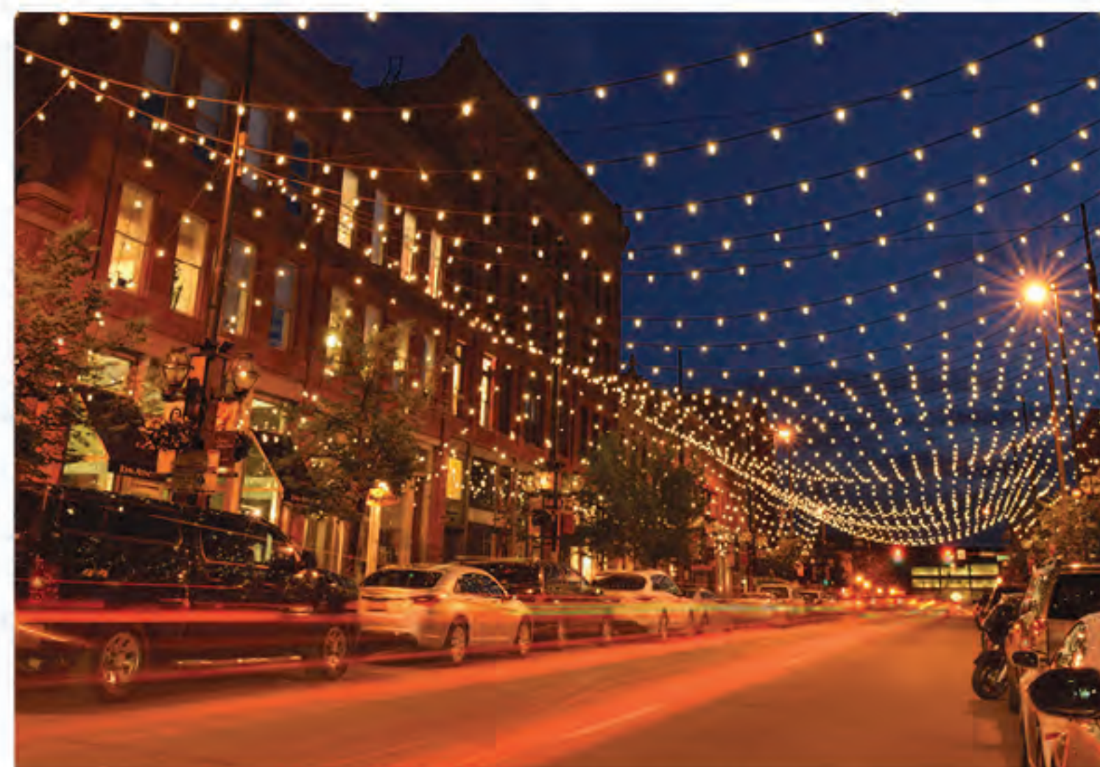
Figure X - Permanent Catenary Lighting(Source)
